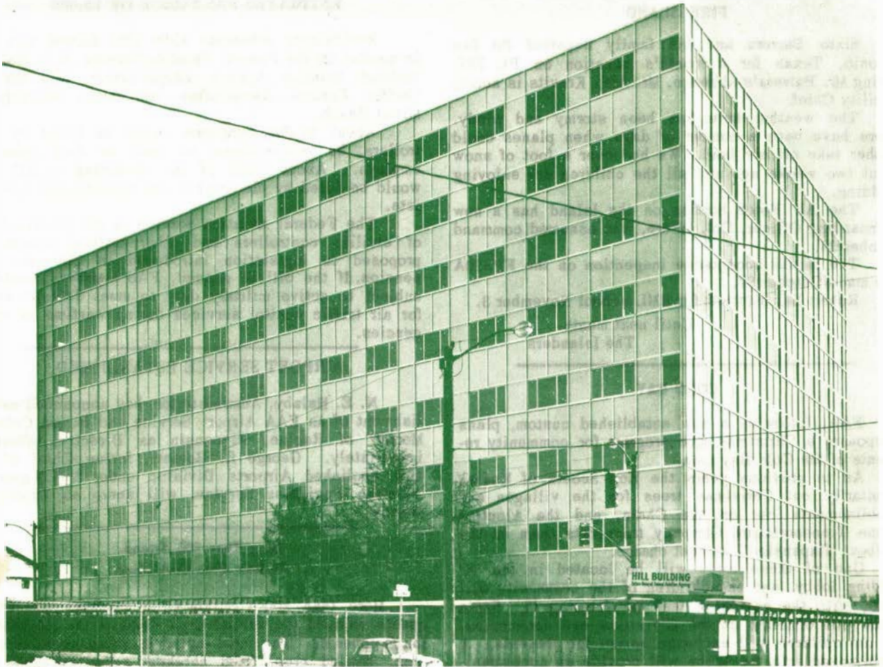
New home for FAA's Alaskan Region headquarters takes shape at Sixth and G streets in Anchorage. Metal panel siding has been completed and workmen are now en-
