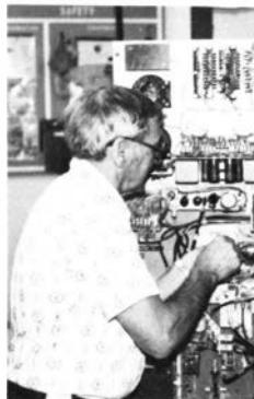
Des Moines navaid technician Einer Jensen maintains one of the 12 VORTACs scattered throughout the sector.
