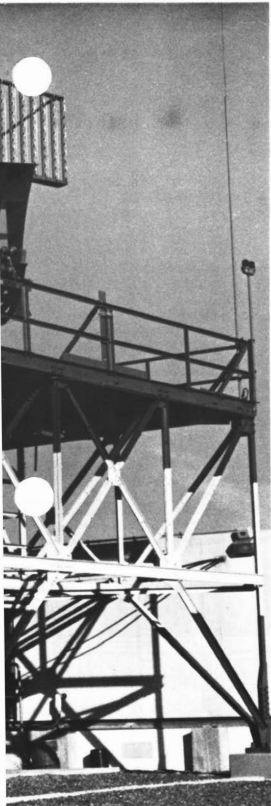
Reno International Airport's surveillance radar dwarfs the sector's Radar/Communications Unit chief Jim Freeman.
