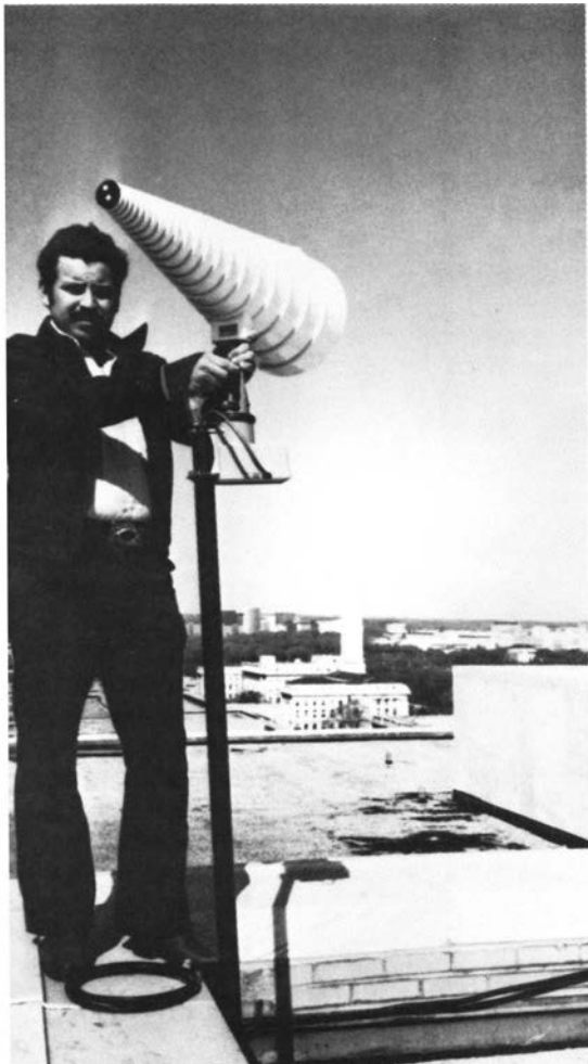
ET Paul Baker installs a conical log-spiral antenna on the roof of the FAA headquarters building. It's used to monitor communications interference.
