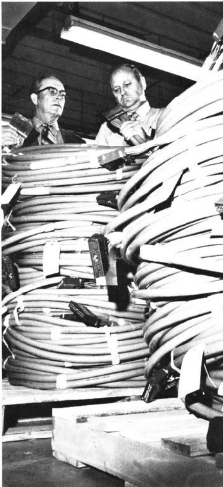
Miles of cables were the sine qua non of automating the en route centers in the early years of the decade. Electronics technicians from all over the country descended on the Oakland ARTCC's future computer complex.
