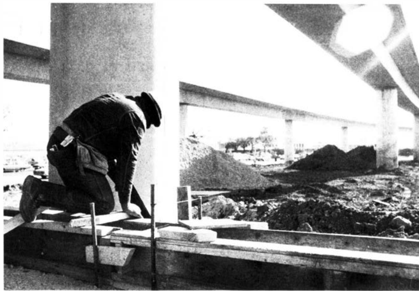
A Metro worker builds a concrete form at the base of the railway's pillared superstructure. The main terminal and airport control tower can be seen in the distance.
