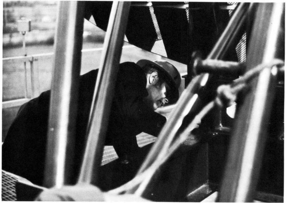
With hardhat and wrench, Detroit AF Sector chief Daniel Reid pitches in for the installation of a new ASR-8 antenna.
