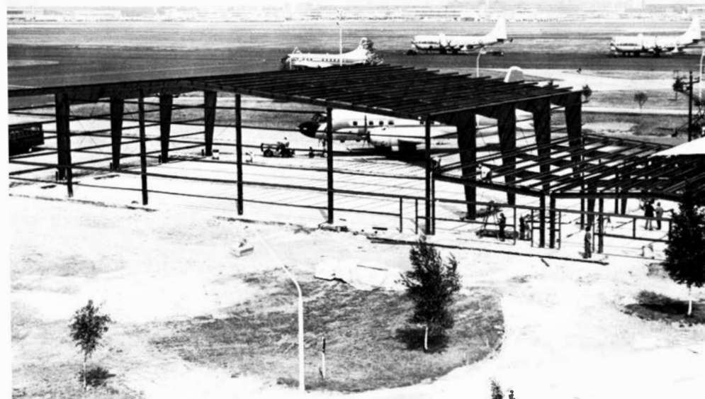
Rhein AFB at Frankfurt shares the airport with the civil aviation terminal (background). In the foreground is a hangar maintenance facility under construction.
