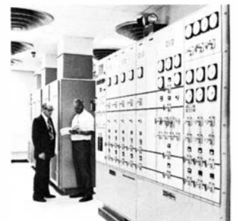
Jim Phennicie, Environmental Support Unit chief at the Los Angeles Center, and his assistant, Rex Shull, check the performance records of the newly installed Power Conditioning System after a local power outage.
