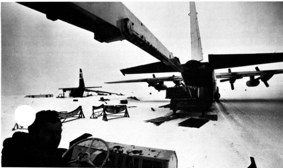
Art Walker operates a crane unloading an airlifted wing section. At left in the background is the damaged plane.
