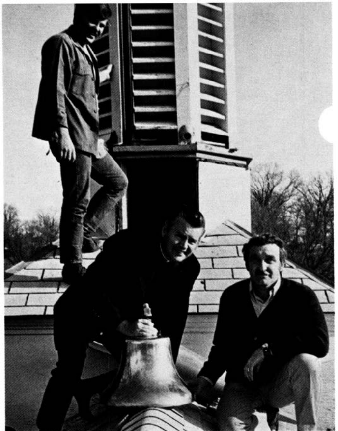
Harrison, Ark., FSS specialist Walter Mayberry kneels on the roof of St. John's Episcopal Church with priest Jim Petersen and a 122-pound Liberty ship bell Mayberry obtained, as carpenter Hank Rogers waits to install it.
