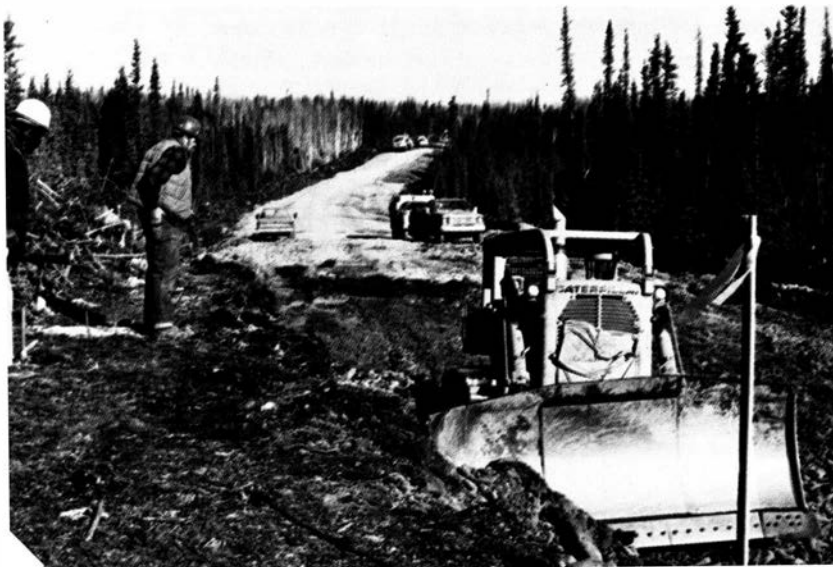
A northern section of the 360-mile pipeline service road takes shape. It will link up with existing roads south of the Yukon.
