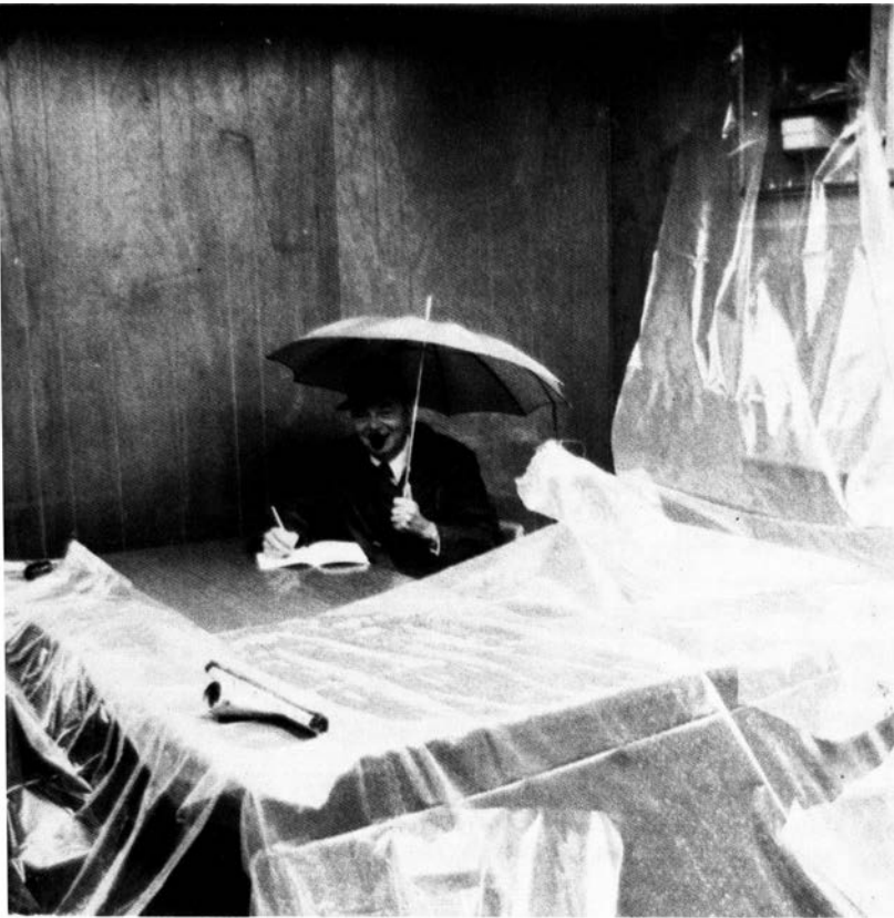
WOULDN'T YOU KNOW IT — Shimmering plastic protects his furniture as Southwestern Region Plans and Programs Branch chief Glenn Compton tries to get some work done. Just when the roof was off during reroofing, Fort Worth got two inches of rain in an hour. It didn't bother Compton much, though; it was his last week before retirement.
