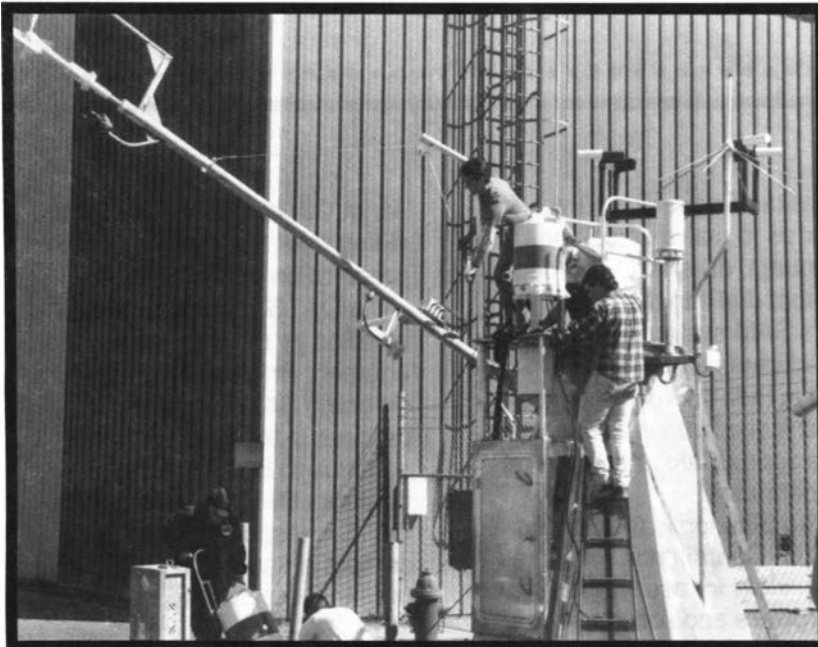
Workers at Reeve rotate the tower down to change out a defective piece of equipment.
